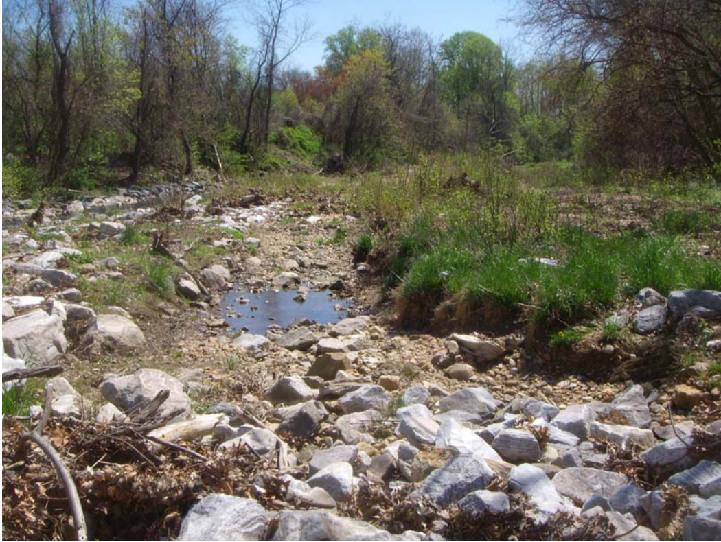
Sligo Creek 1 – scour channel along right bar, April 2008
