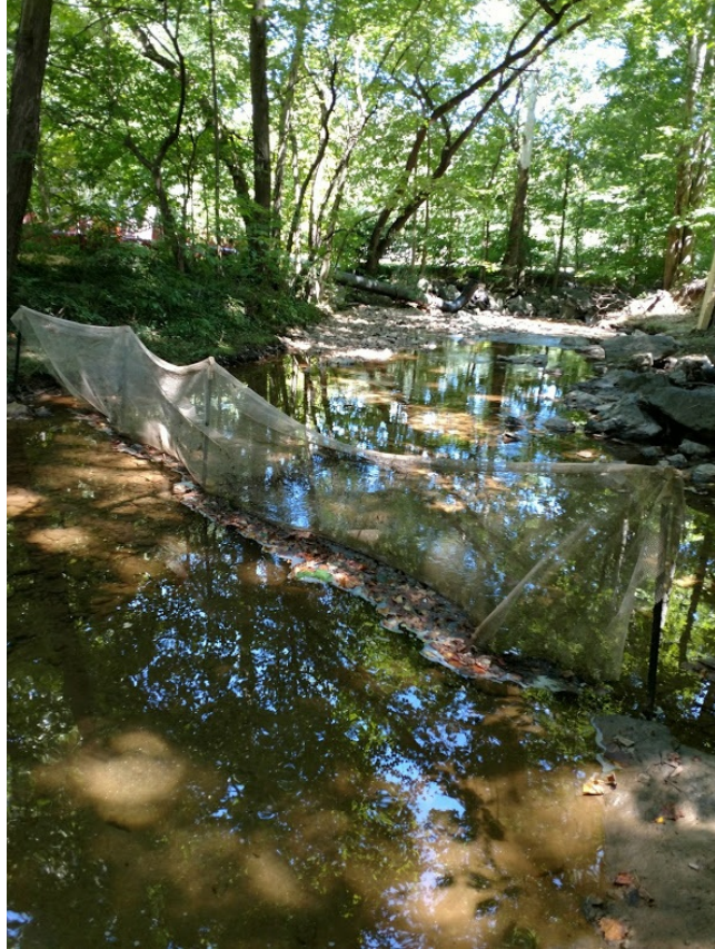
Netting across Sligo will keep fish from work areas during stream bed restoration.
