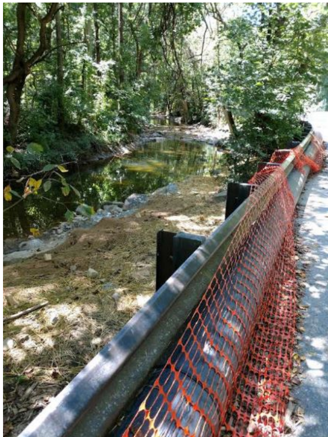
Black plastic pipes will divert creek water around the restoration site during the work. (Wilpers photos)
