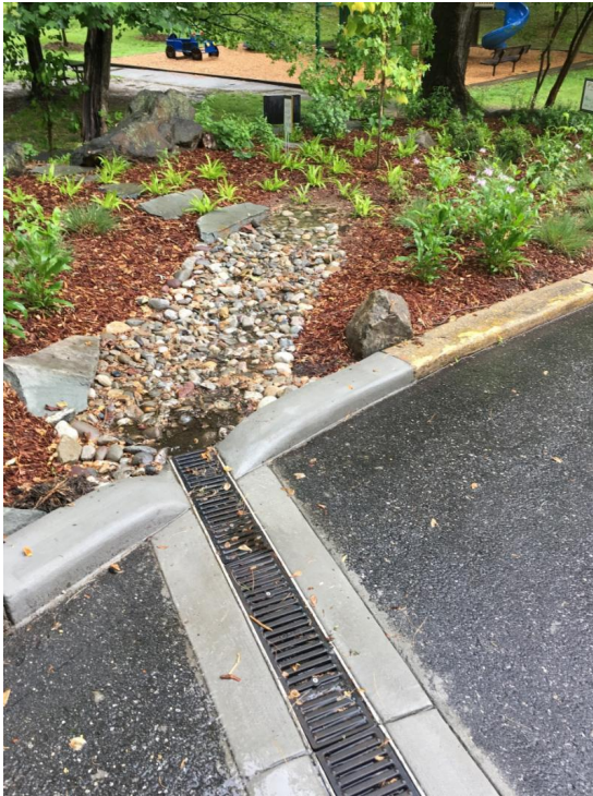
A portion of the new stormwater management project in the Three Oaks neighborhood (M. Harrell photo)
